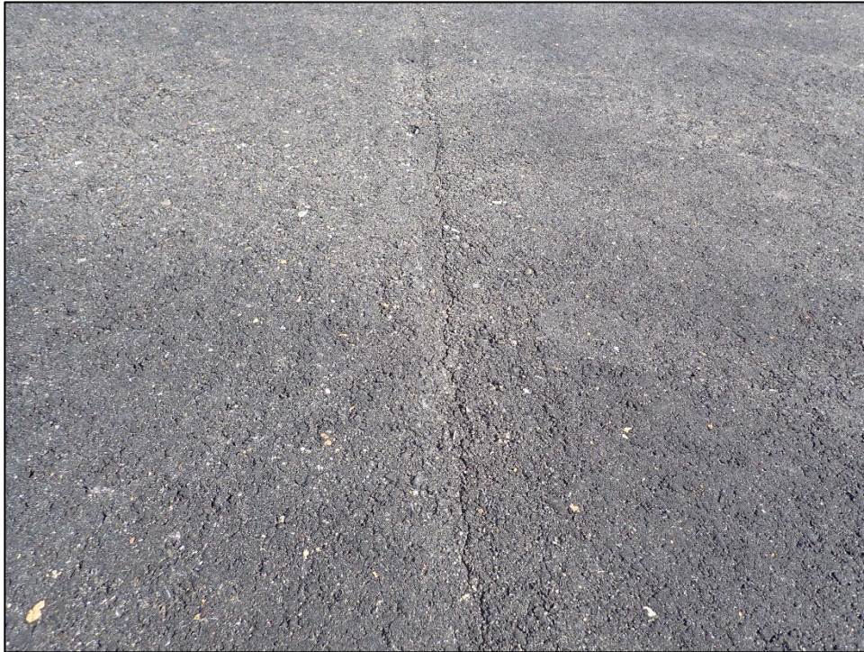
AP-03-10: L&T Cracking
