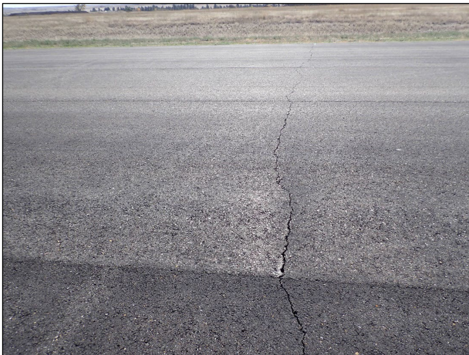
RW09-11-64: L&T Cracking
