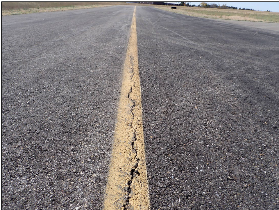
TW-13-04: L&T Cracking
